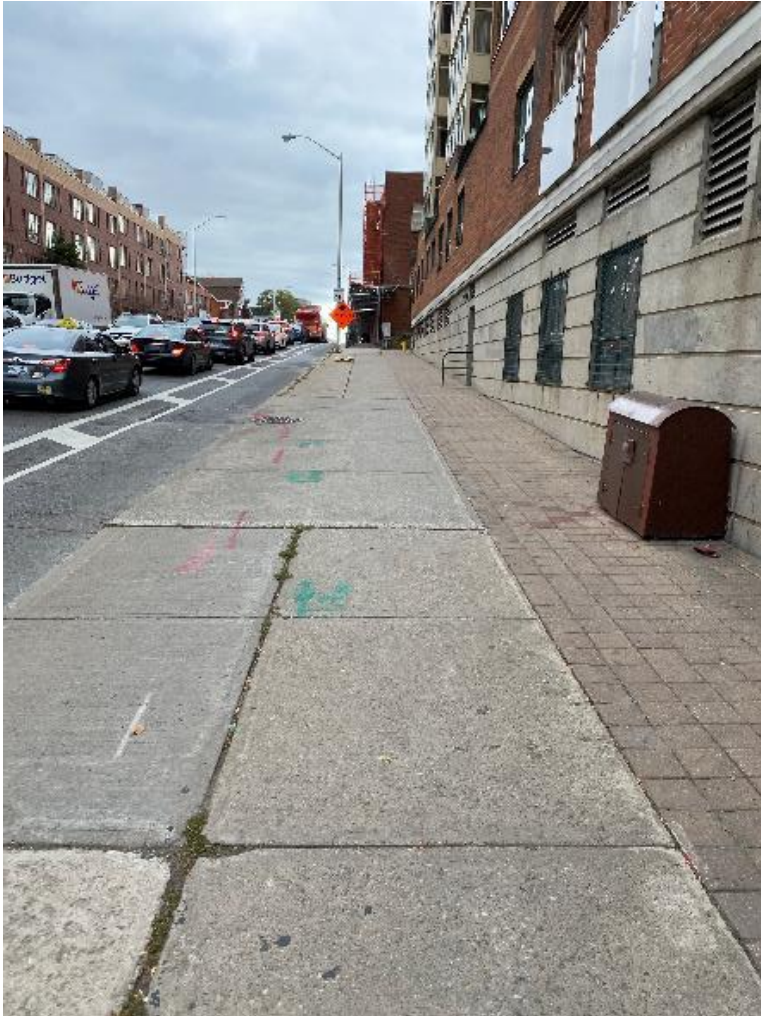
Sidewalk condition along north side of Bloor St W
