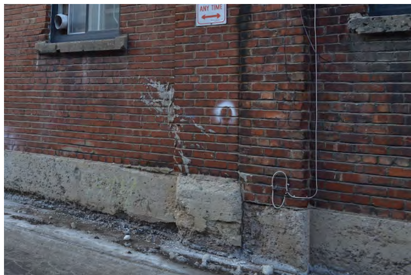
Building C south elevation, showing joint between two construction phases, severely weathered and damaged foundations, cracked and chipping stone sill, see photo to the right for larger context.
