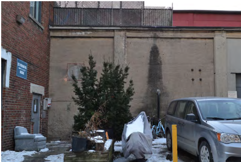
Building B (west) east elevation, showing interrupted bay adjacent to Building B (east), localized surface staining, and new red cladding at clerestory window.
