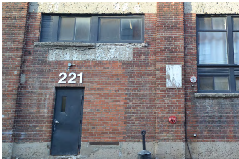
Building C (east) south elevation, showing brick infill at original service door opening.
