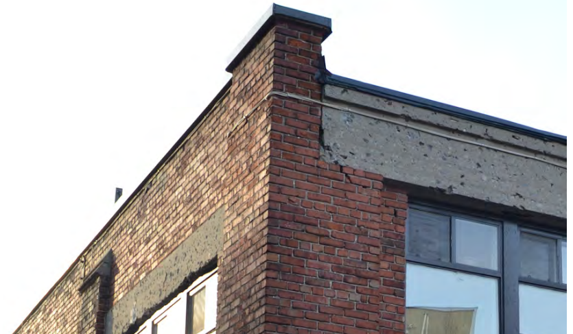
Building C (east) south-east corner, showing large crack and weathered condition of parapet.
