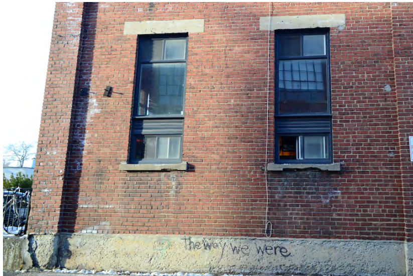
Building C (west) south elevation, showing weathered condition of brick wall, window sills and lintels, and concrete foundation.
