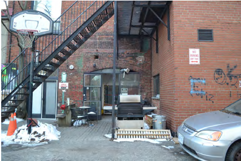
Building A east elevation, showing ground level four-tier segmental arch doorway and miscellaneous staining damages to the brick face.
