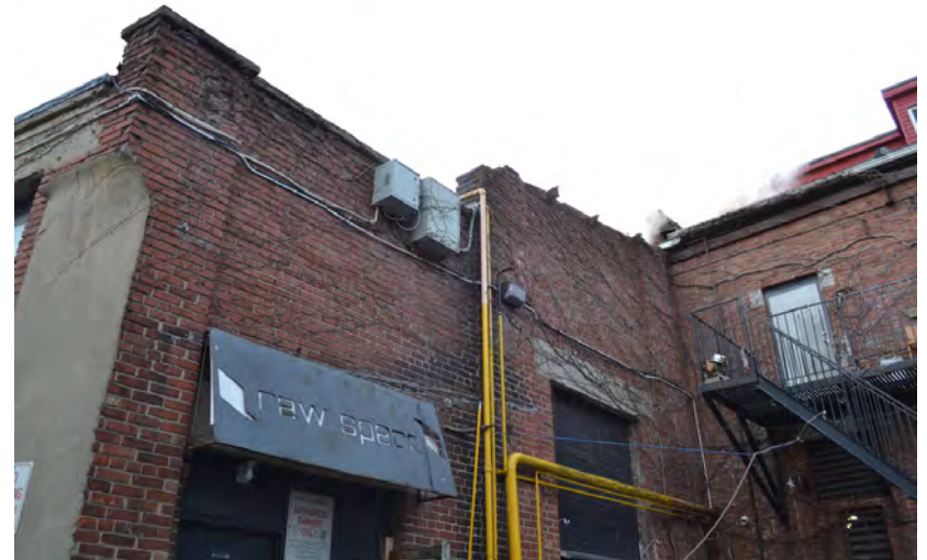
Building C (east) north elevation, showing two original service door openings with new infills, vestiges of a removed steel frame covered roof structure at Building B (east), and the removed brick pilaster of east elevation now parged.
